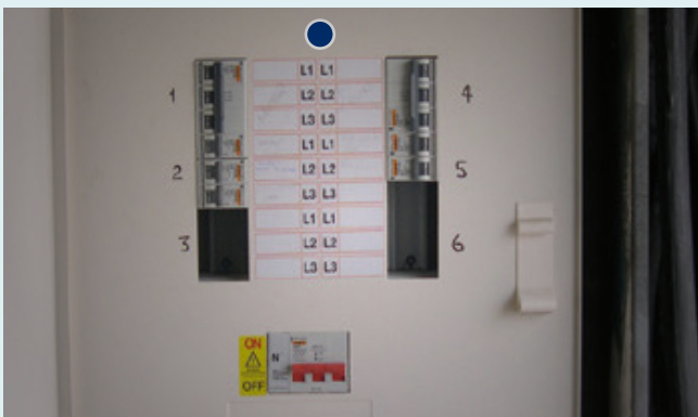
Secondary Distribution Board
